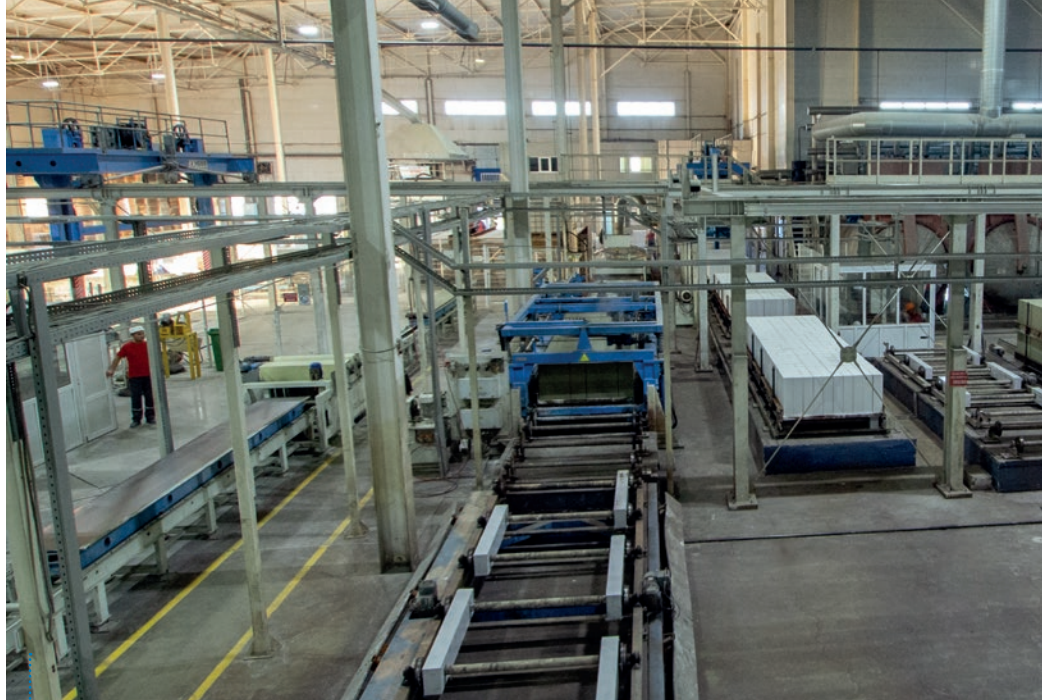
View into the production hall with tilting system for cut green cake (left) and autoclaves (right)
