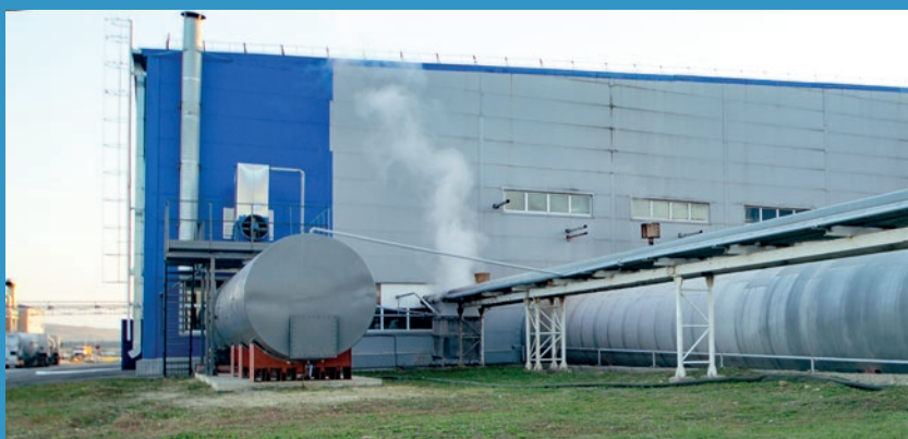
Container and plant for collecting, cleaning, and reuse of the condensate derived from the autoclaving process. The equipment was designed and built by members of DSK Gras-Svetlograd’s own staff.
